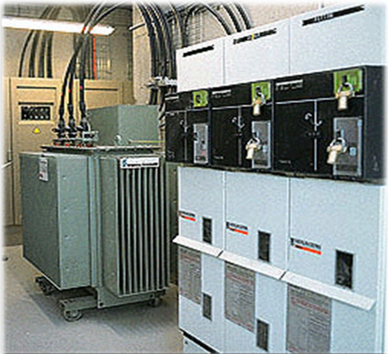
Figure II.3: poste de transformation 30kv. .[2]
