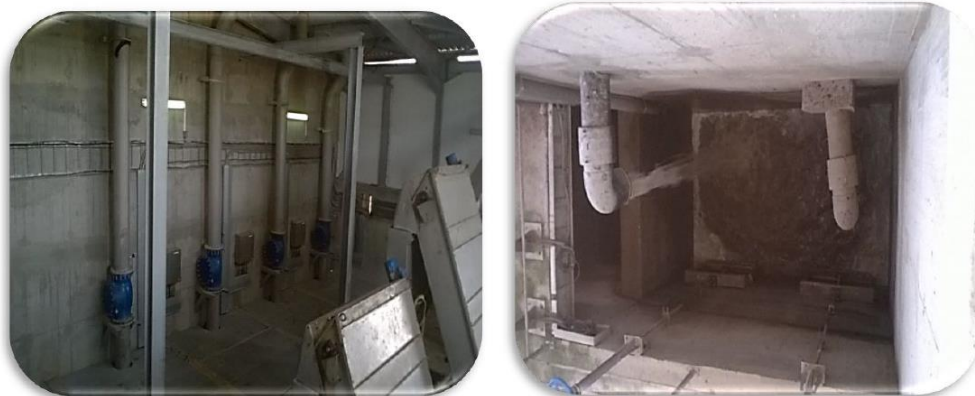
Figure II.6 : Pompe de relevage
