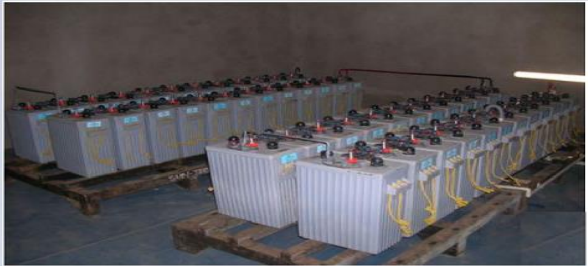
Fig.II.14. Location of battery bank in a separate well ventilated room [7]
