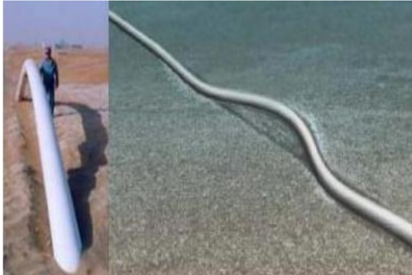
Figure III. 3: Dommages mécaniques (ondulation) [16]
