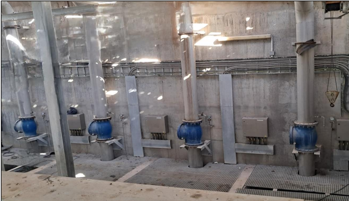
Figure 10. Pompes de relevage (2024)
