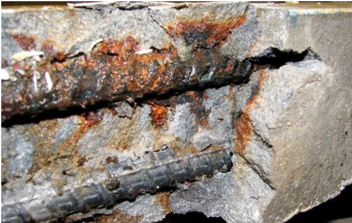
Figure 2-3: Corrosion des armatures 4
