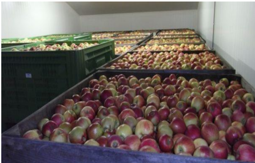
Figure II.7. Refrigeration and Storage
