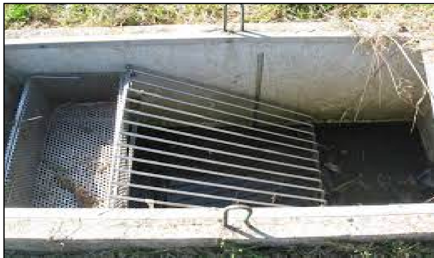
Figure II.6: Grilles à nettoyage manuel
