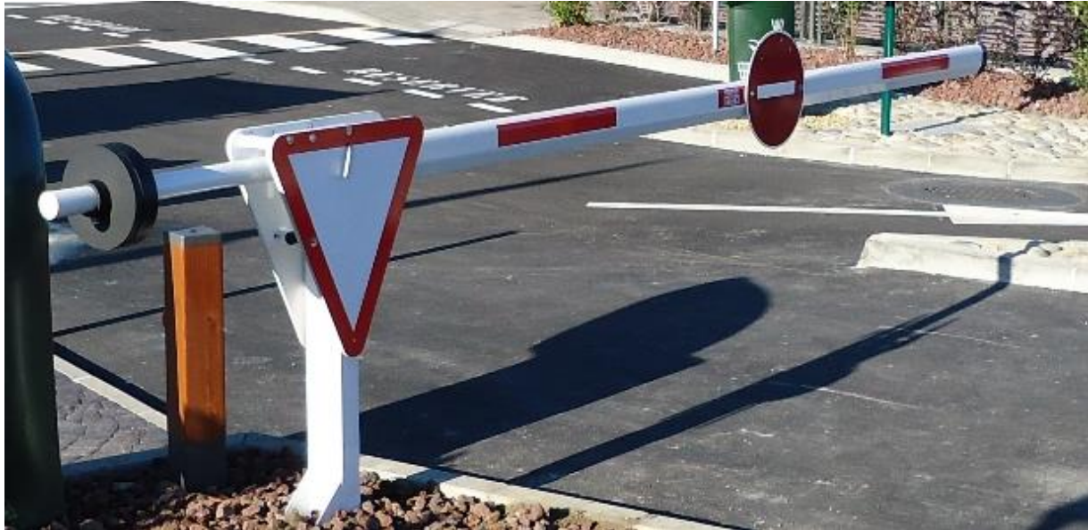
Pic 2..... BML lifting manual barrier
