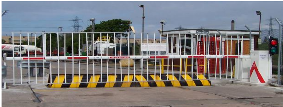
Pic 11..... HB lifting barrier
